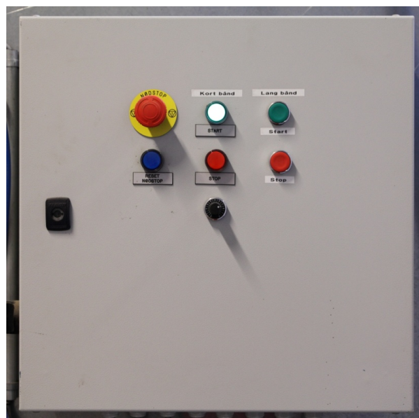
Figure 10: Front of the electronics cabinet placed on the RDF-Sorter
