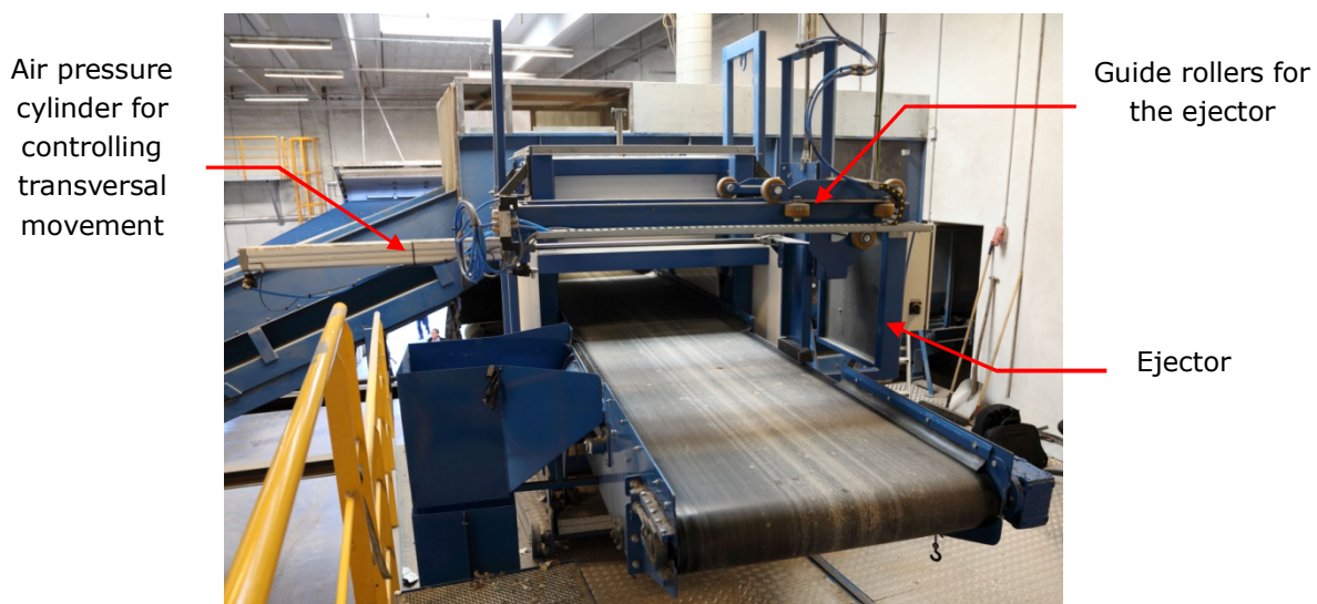
Figure 21: RDF-Sorter installed at nomi i/s
