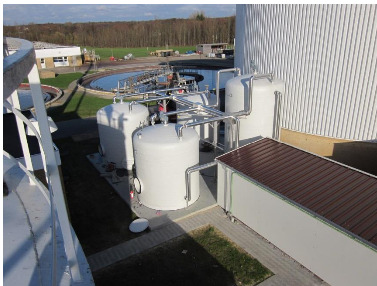
Hydrolysis plant including engineering building. Photo Niels Oestergaard
