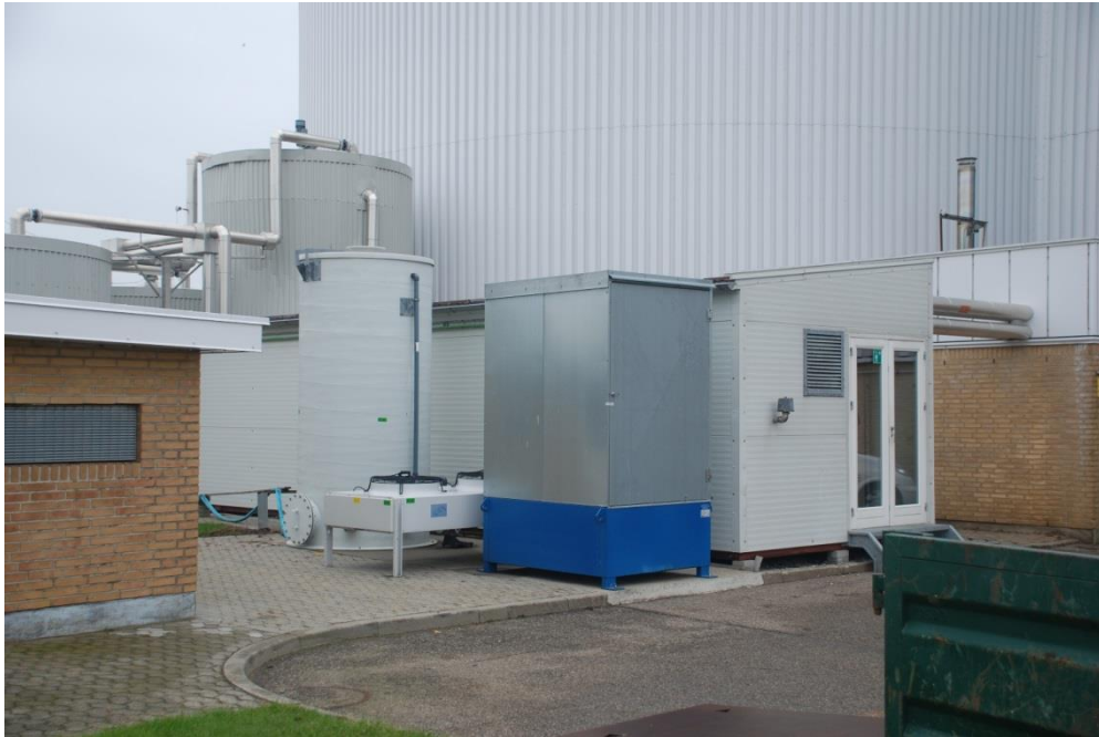
Odour gas scrubber including acid cabinet. Photo Niels Oestergaard
