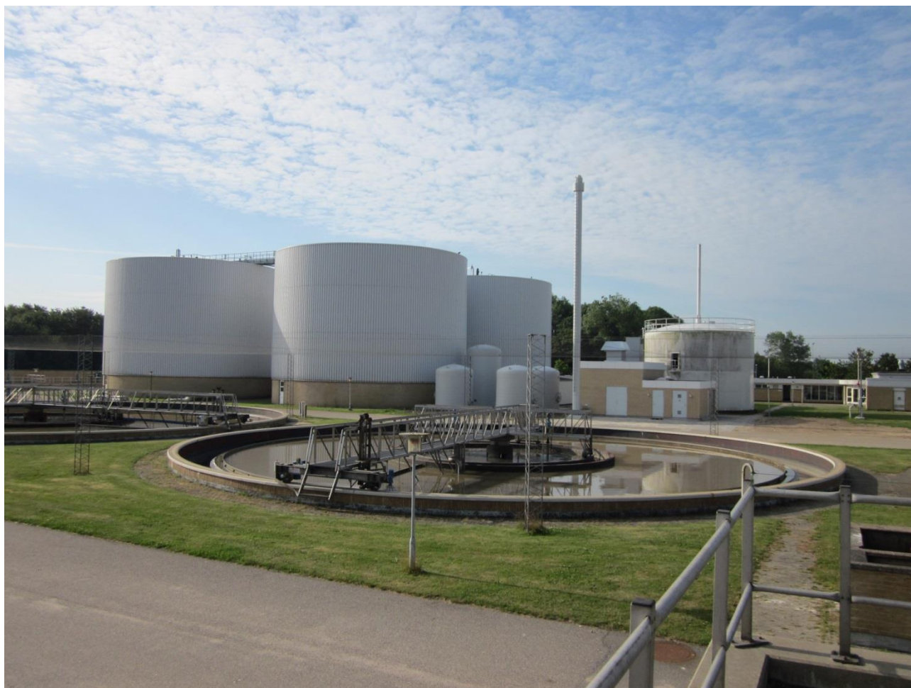
The relative small hydrolysis tanks in the middle. Digesters at left. Photo Niels Oestergaard
