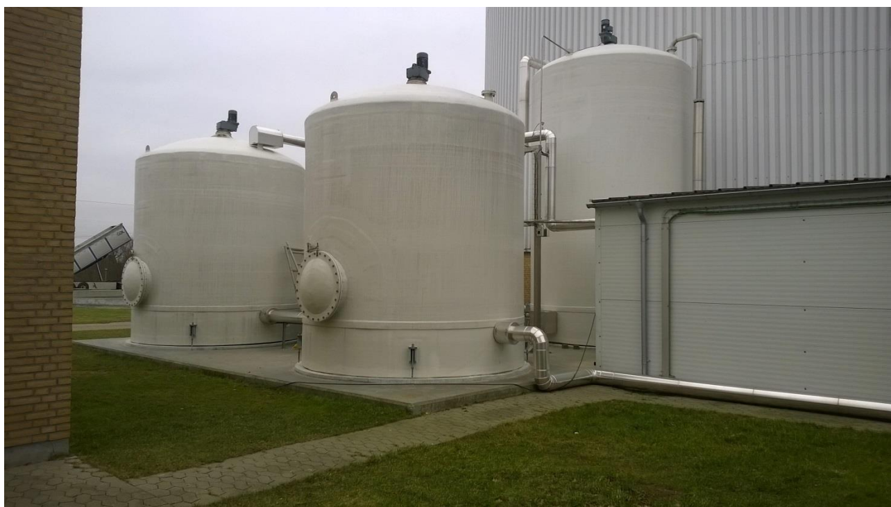
New hydrolysis tanks and simplified gas system after rebuilding the plant. Photo Niels Oestergaard
