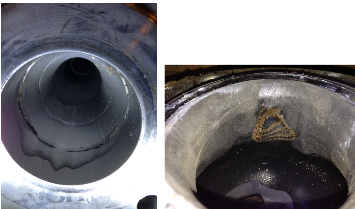
Figure 12. Wear on parts of the equipment was evident. The wear is caused by the sand in the feeding stream. Left: Flash-out out-coning pipe. Right: Compensator on the flash out pipe.
