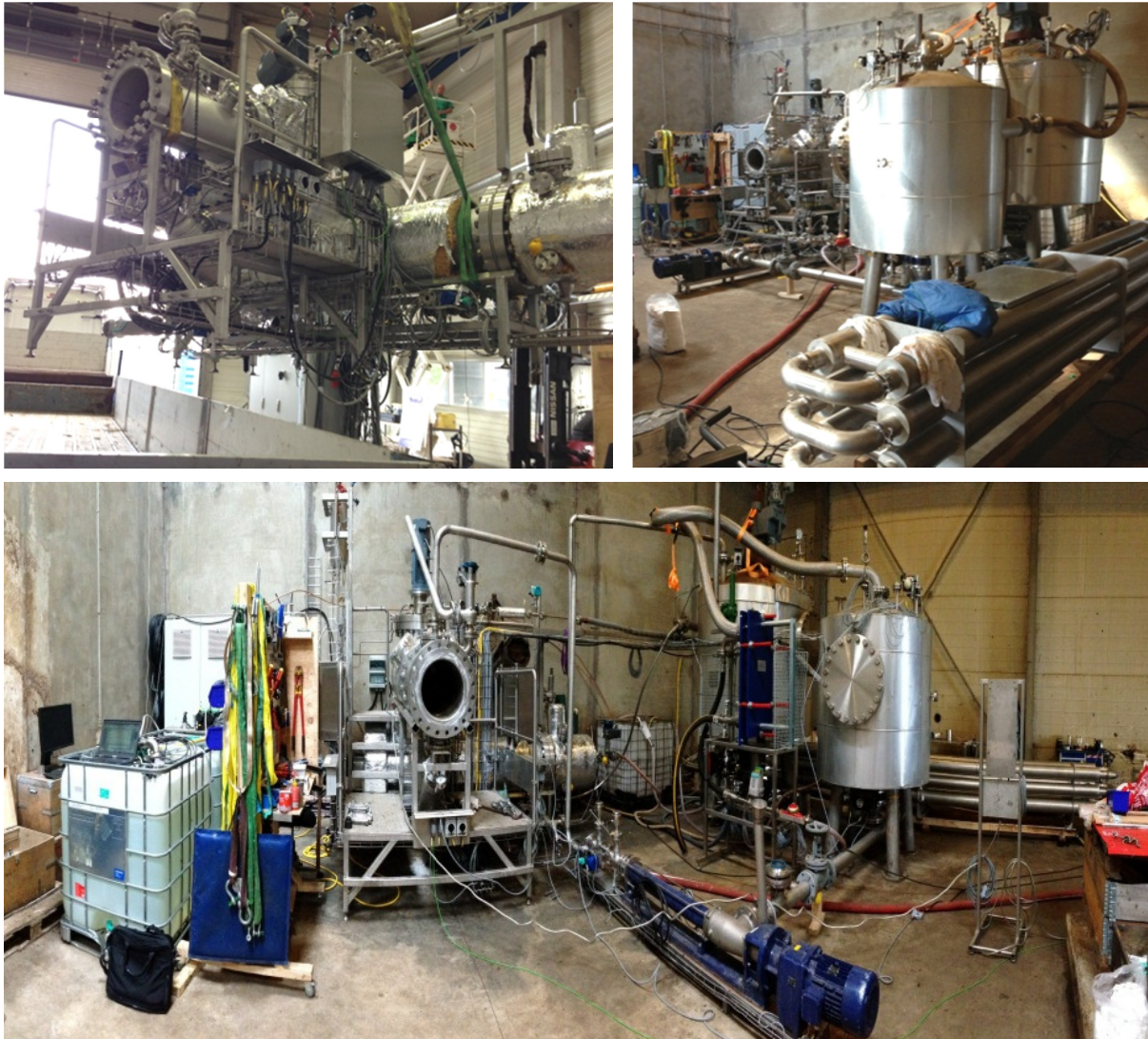
Figure 6. Implementation of the unit at Biokaft's biogas plant, July 2013. Arrival of the Carbofrac® unit (top left), installed Carbofrac® unit with auxiliary equipment such as tanks and the mono-tube heat exchanger (top right) and the whole installation (bottom). At the time of the pictures dewatering trials were still ongoing and therefore no screw press is present.
