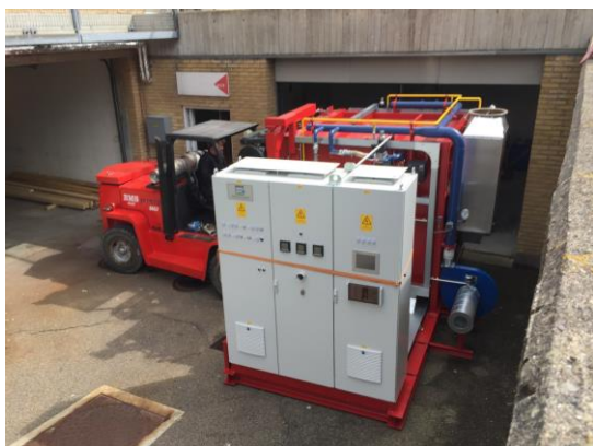
Fig. 5a: A forklift with a lifting capacity of 5 tonnes was used to transport the pilot plant from truck to final placement in a basement under the DTI.
