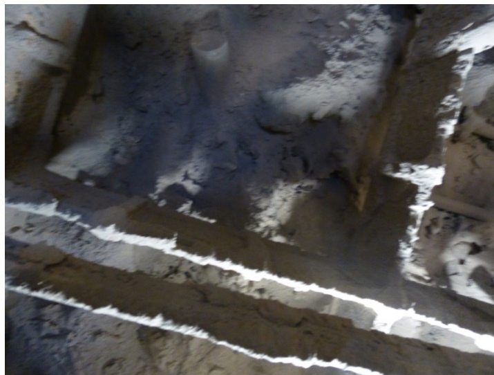
Picture 1 Close up picture showing the first catalyst tray in first bed (upper bed) seen from above, all monoliths and tubing are covered by dust /slags thus obstructing the catalyst function
