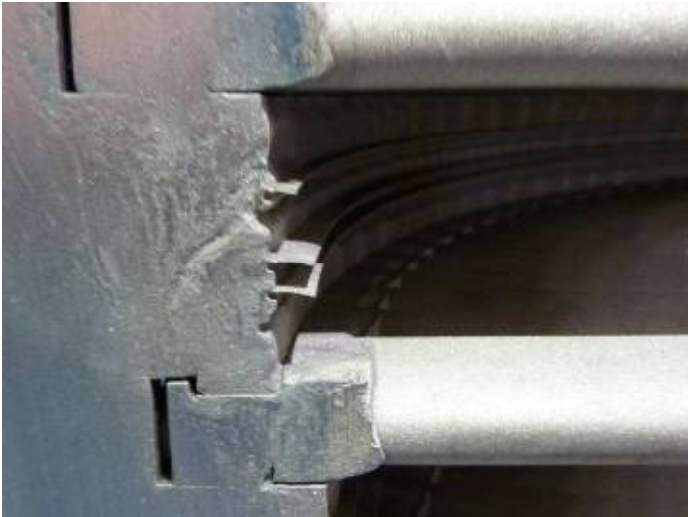
Figur 15. Erosions/korrosions skader "stator carrier rings" i HT turbinen stator-element 42 – 47 [ref. Siemens].
