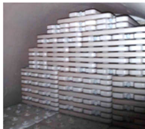
Storage bricks of phase change material (SINTEF Energy Research)
