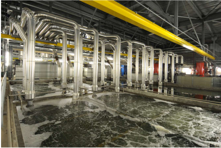
Fig. 3.1. Ice storage tanks (Source: www.enertherm.fr ).
