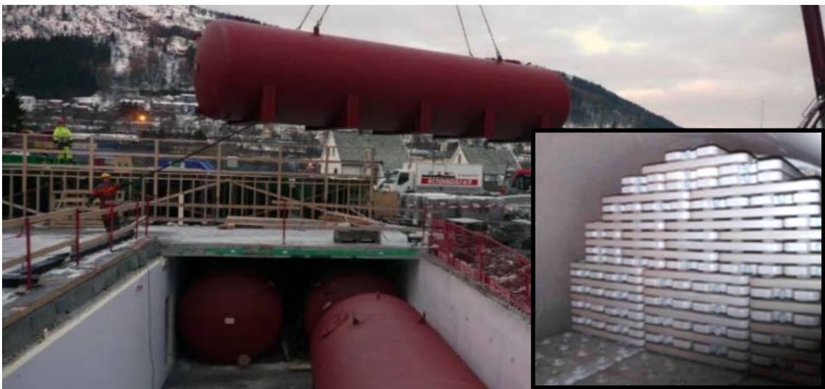
Fig. 3.8. PCM tanks for cold thermal energy storage at the University College of Bergen, Norway [27].
