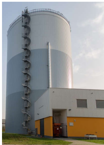
Fig. 2.7. Thermal energy storage district heating system Potsdam, Germany [13].
