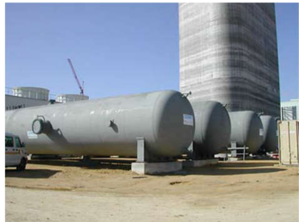
Fig. 4.11. Steam accumulators installed at PS10 in Spain (© Abengoa Solar).
