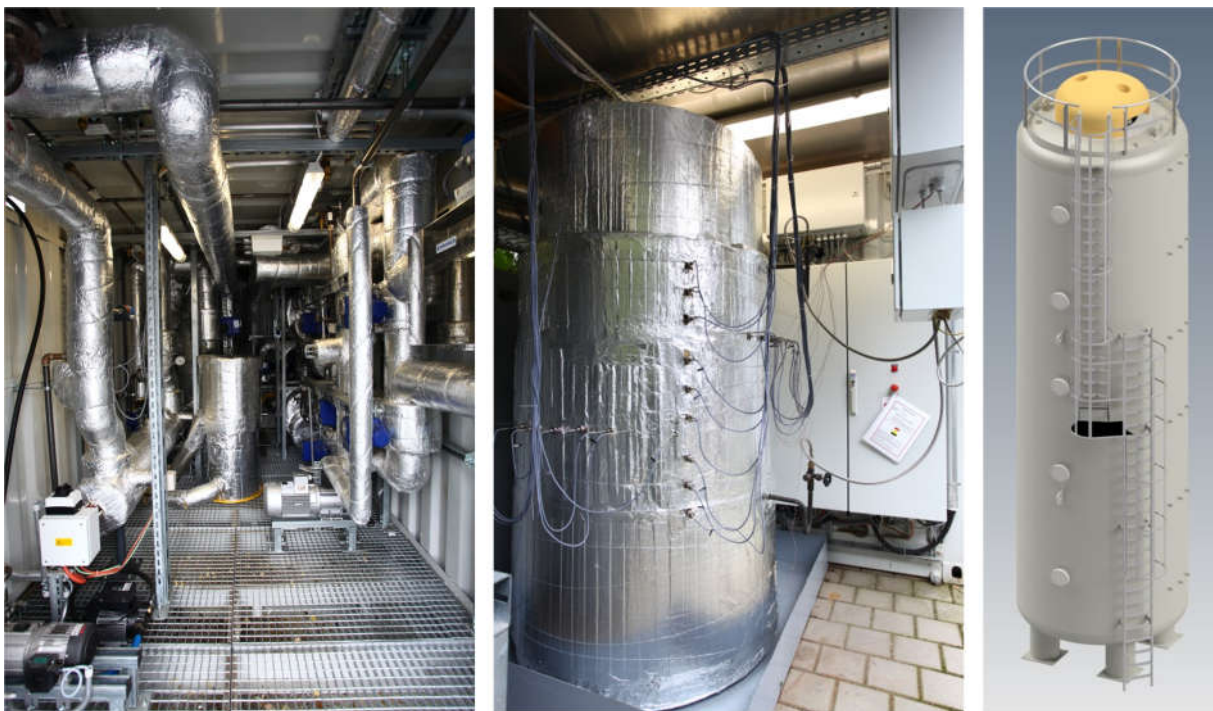
Fig. 4.16. Thermal energy storage test site at ZAE Bayern, Garching.
