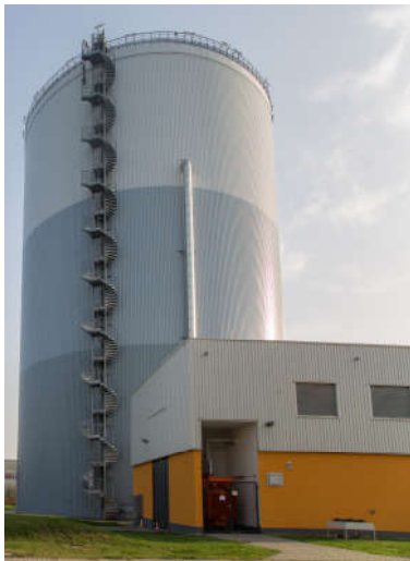
Hot water storage in Potsdam, Germany (City of Potsdam)
