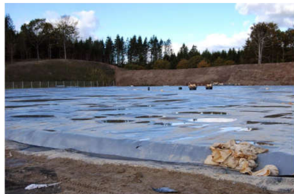
Fig. 2.4. Pit storage with floating cover.
