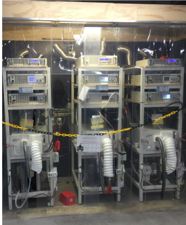
Fig 45 – air cooling pump
