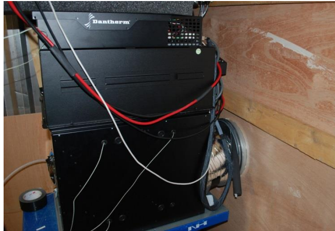
Figure 19: Illustration of the climate kit installed in the climate chamber. The system is installed in a temperature of about 10 degrees Celsius, drawing intake air from the cooling container at about -32 degrees Celsius.
