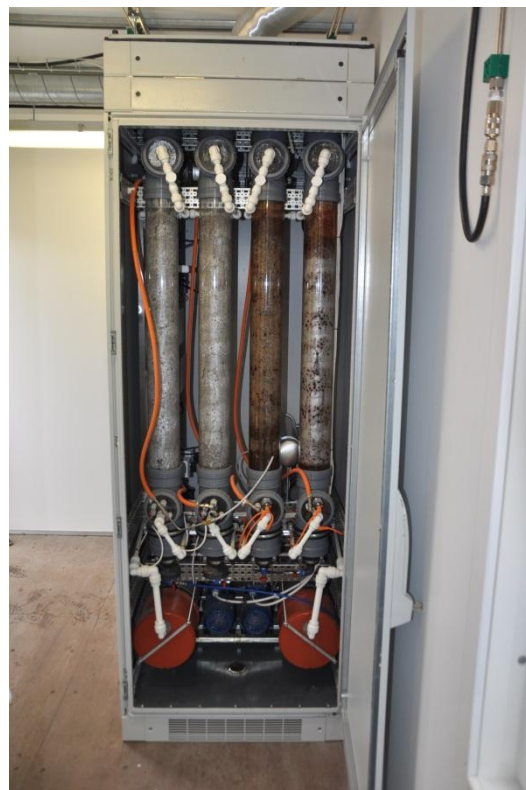
Picture 1 Cleaning unit.
