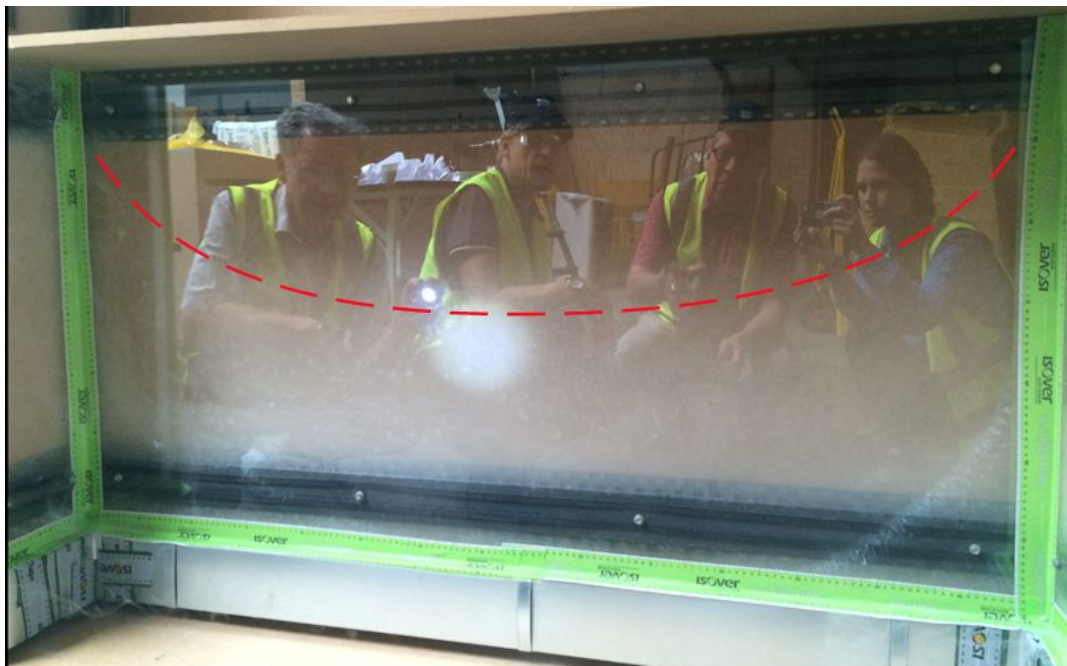
Figure 48: Movement of air beneath window visualized with smoke test
