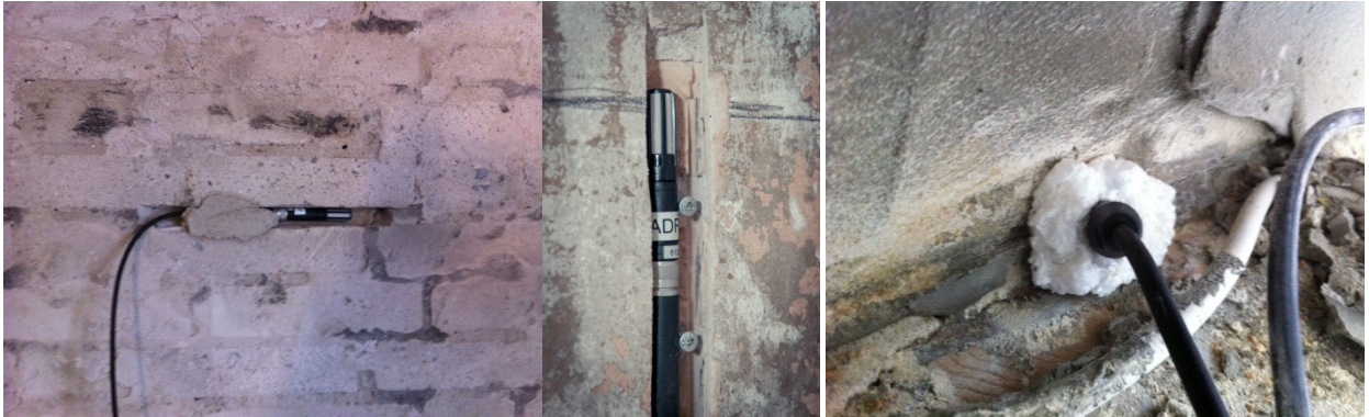
Figure 2: Sensors placed (from left to right) in existing joint, purposely-designed notch, and drilled to beam end.
