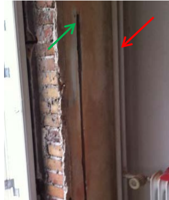
Figure 15: Hot water pipes (red arrow) in the vicinity of sensor 6 location (green arrow)
