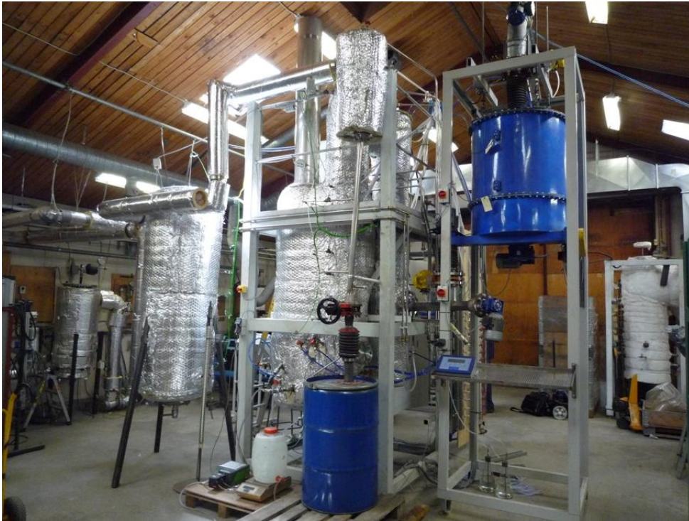
Figure 3: 100kW test plant at DTU
