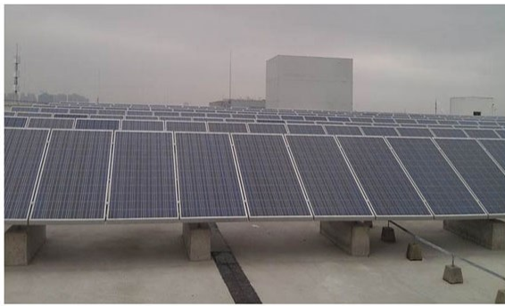
Rooftop building photovoltaic installation
