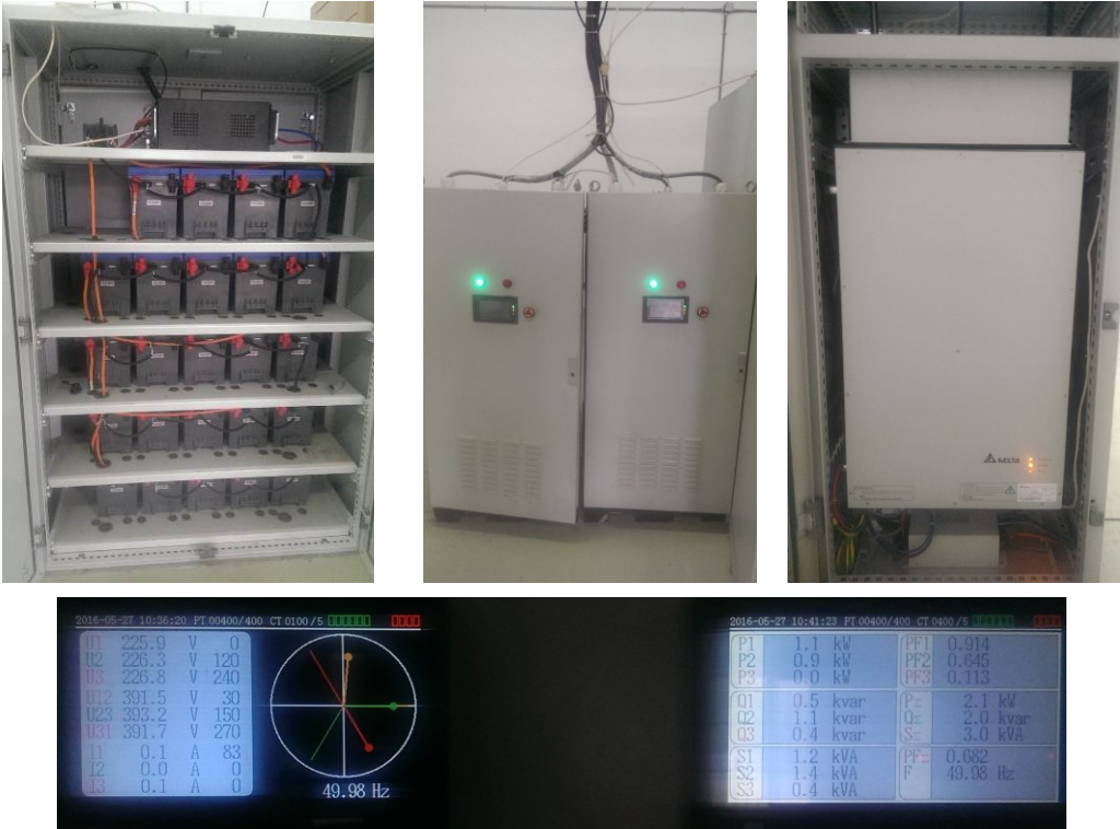
Fig. 17. Test in Shanghai MG site: batteries, power electronic converters and measurement display
