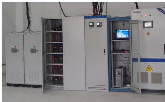
Battery energy storage system, power electronics and control
