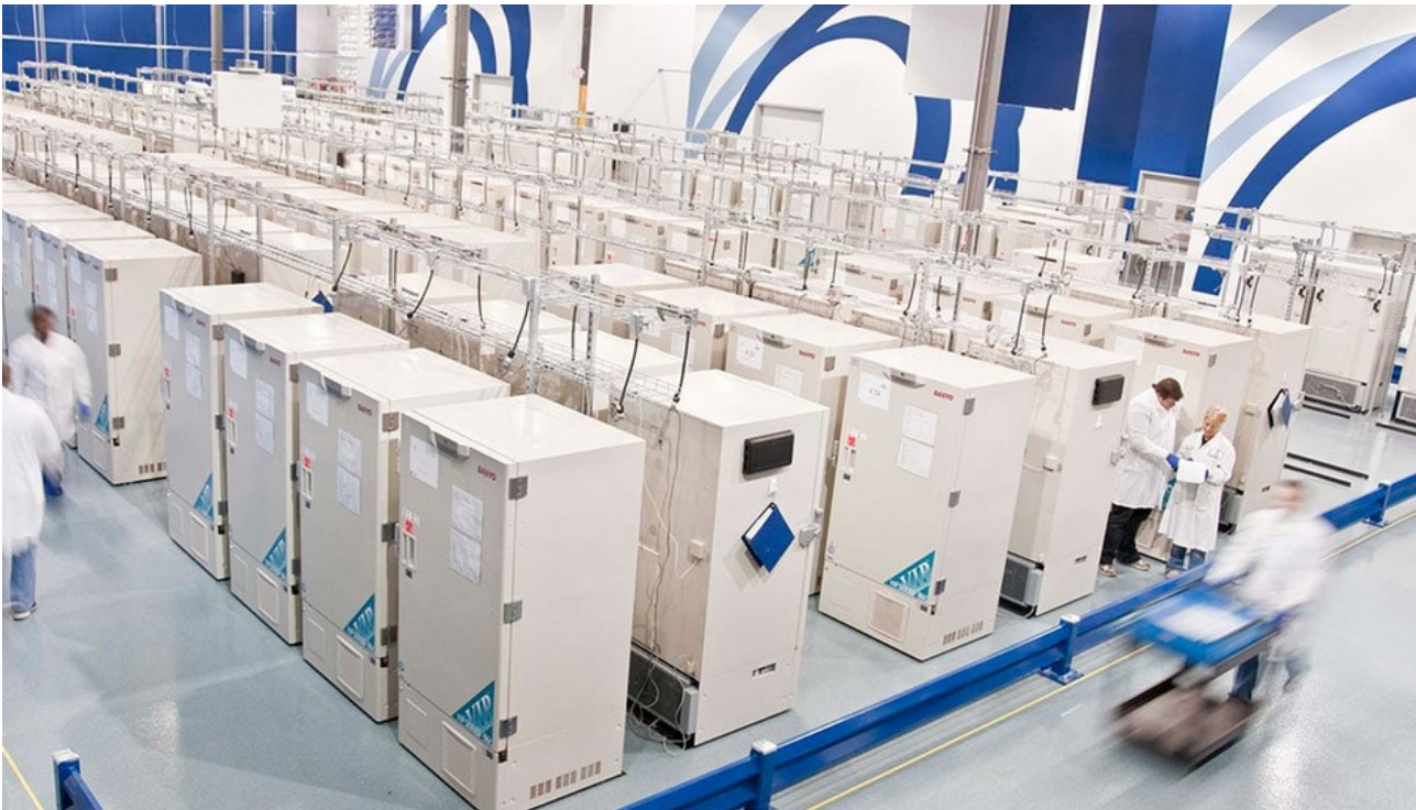
Freezer demand lot of space and energy (picture: Brooks)
