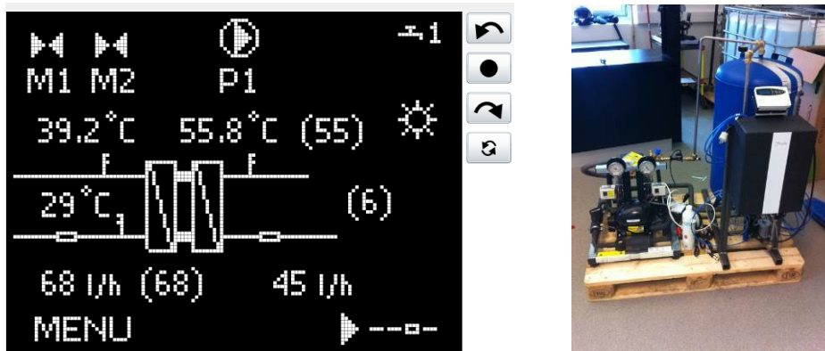
Figure 9: Left: Display of electronic controller, accessed via web portal (ECL portal). Right: System test equipment
