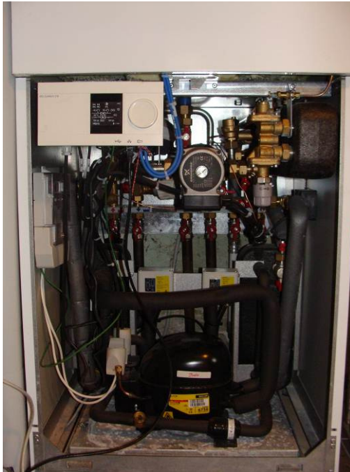
Figure 16: Pictures of one of the low temperature district heating units
