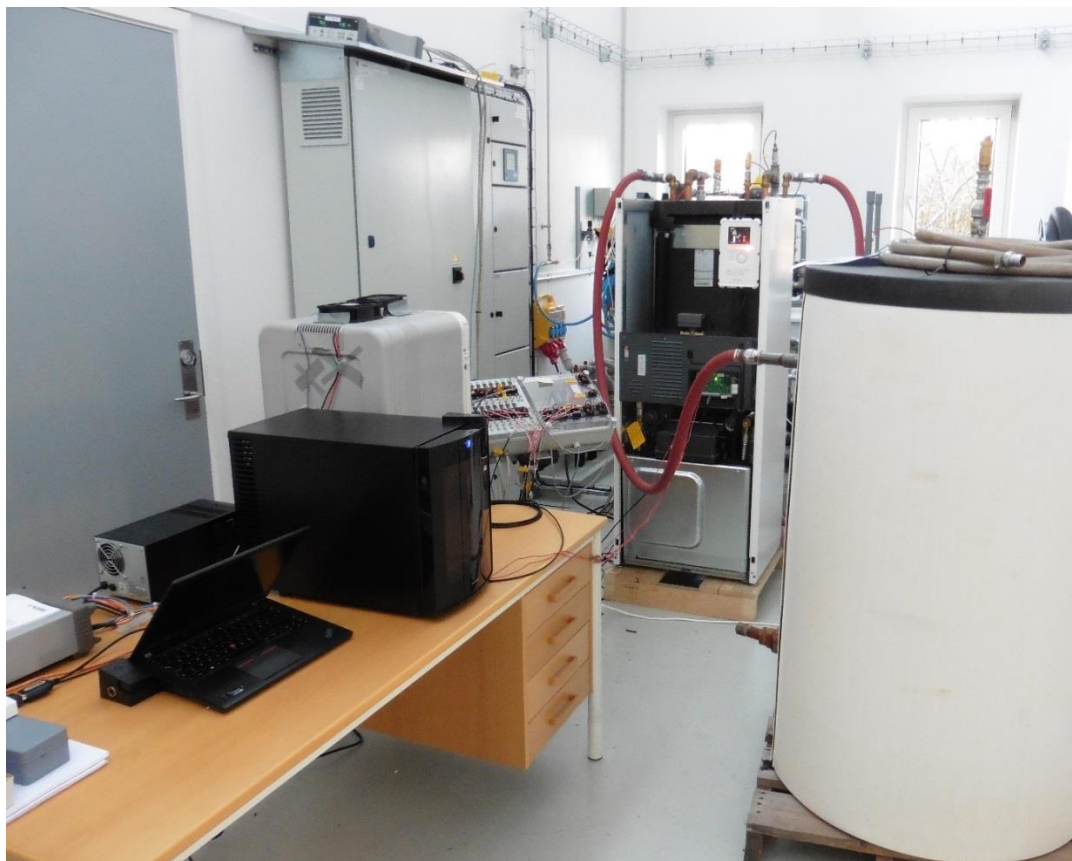
Figure 21 A heat pump installed in the conventional test rig with the additional dynamic test equipment placed on the table. SG Ready and the dynamic house simulation running on the laptop.
