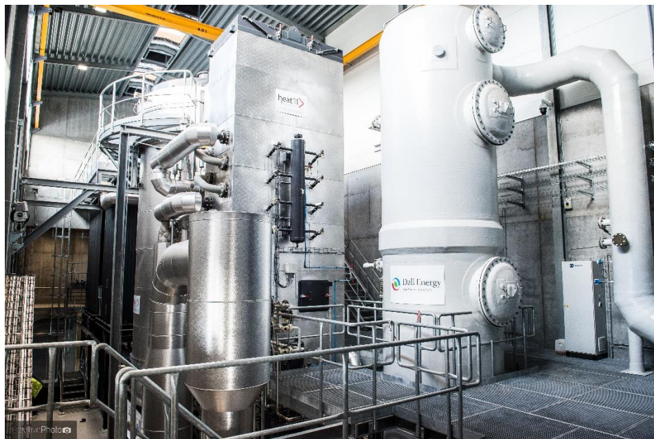
Picture 2 - Main hall at Sindal CHP Biomass Plant
