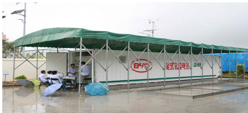
Figure 3.1.9: BYD 800kWh / 200 kW container for bulk storage
