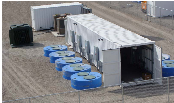
Figure 3.3.3. Photo of Beacon Power flywheel installation in commercial operation in ISO New England, USA, since November 2008. The picture shows 10 flywheel modules lowered into the ground (5 on each side of the container). Source: Beacon Power.
