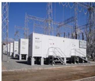
Figure 3.1.5: From A123 Chile installation
