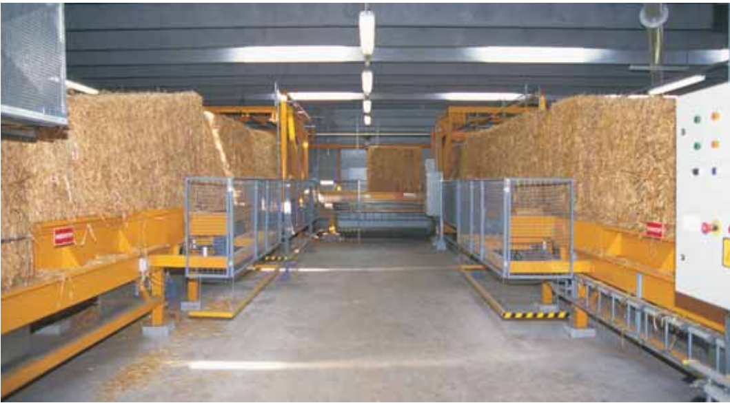
Two of the four feeding lines at Studstrupværket leading the straw from the storage to the shredders.
