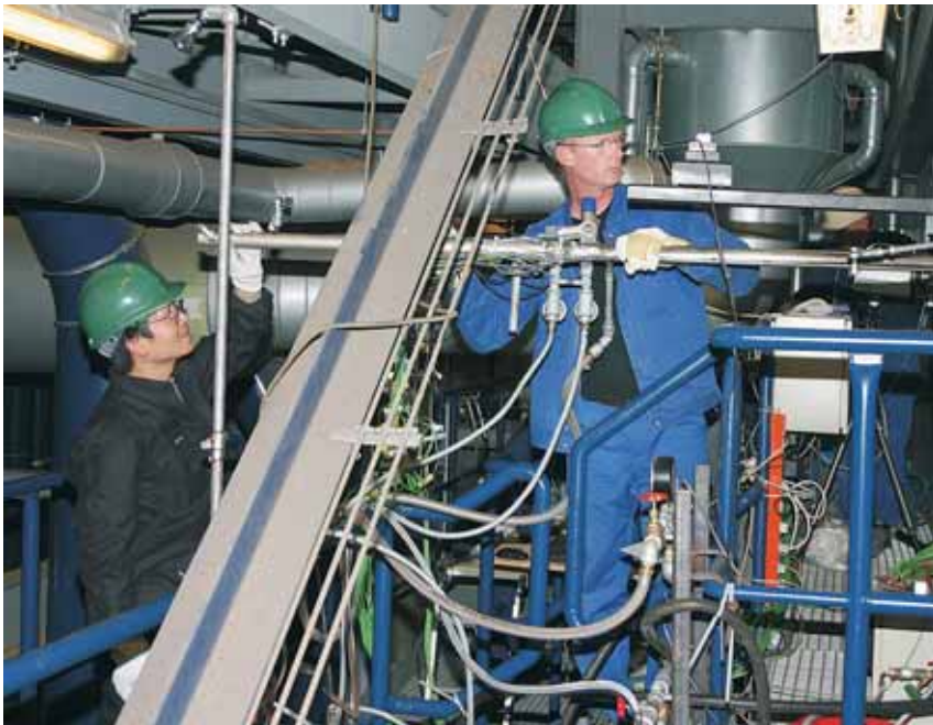
Employees from the CHEC group at the Technical University of Denmark measuring the deposits on a biomass-fired power plant boiler.
