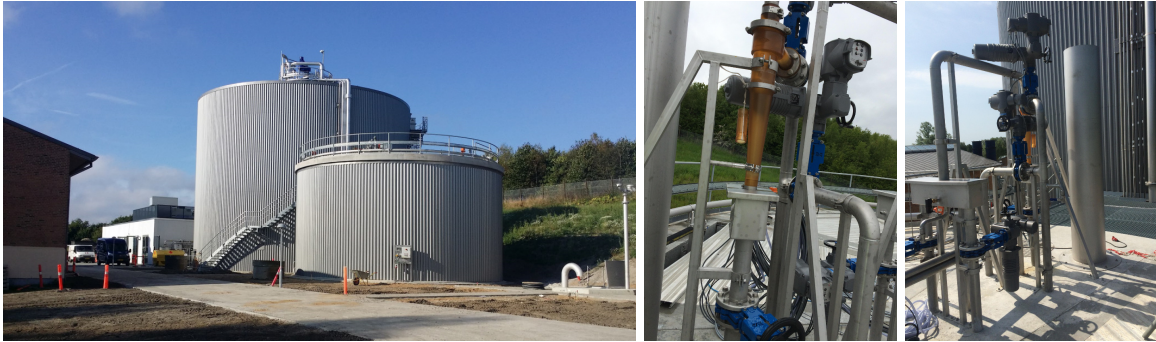
Figure 3: Photo of the DEMON®-tank in front of the digester (left), DEMON® cyclone(middle), Installations at the top of the DEMON® tank (right).
