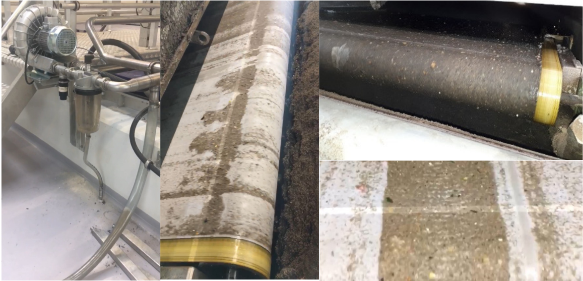
Figure 11: Left: New vacuum suction installation, Mid: Filter mesh without proper build up of sludge Right, top: Filter mesh, which a good build up of sludge Right, bottom: Filter Mesh with stripes, as it looks when the nozzels do not work properly
