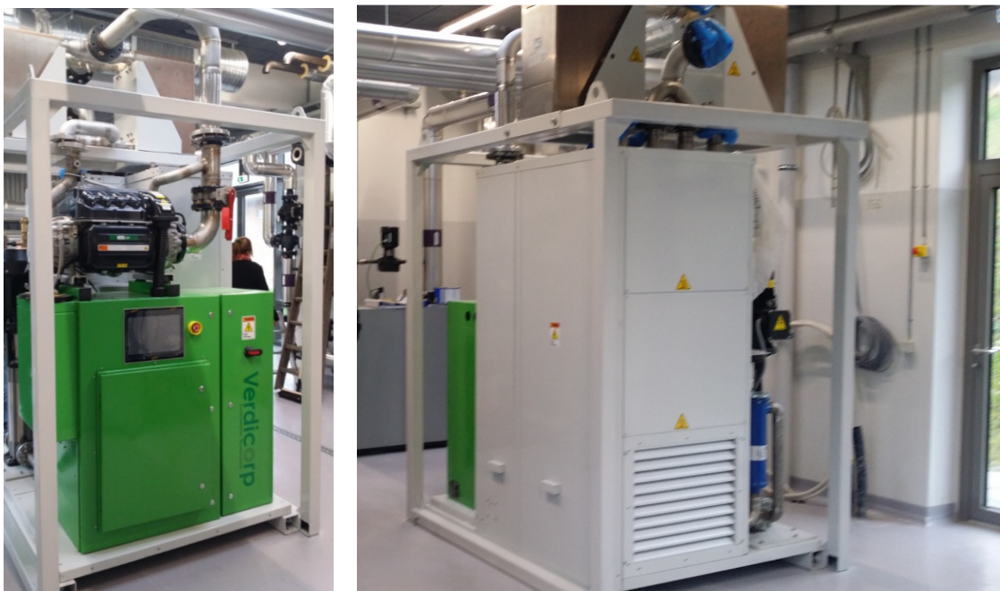
Figure 13: Organic Rankine Cycle (ORC) installed at Egaa WWTP
