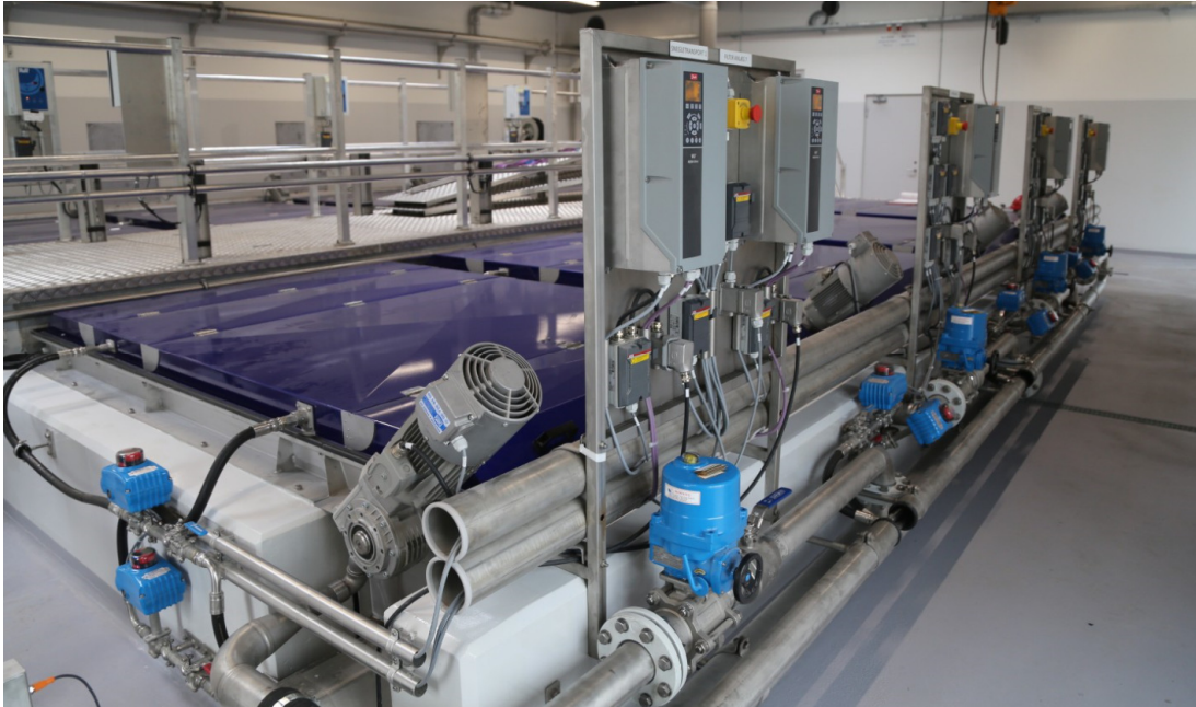
Figure 9: Salsnes filters installed at Egaa WWTP
