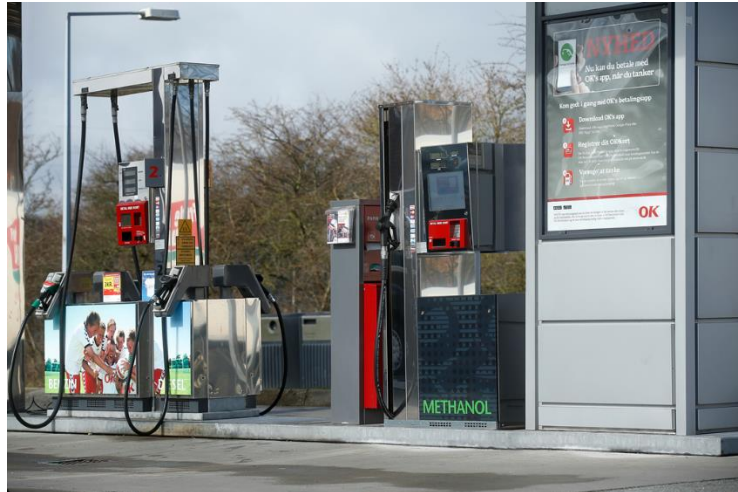
Skalborg Methanol Mix Refuelling Station
