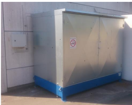
External Methanol Fuel Mix tank
