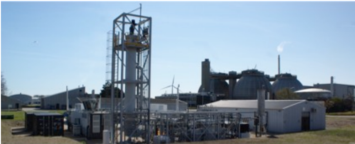
Figure 1.1 Photograph of P2G BioCat Plant on BIOFOS site in Avedøre, Kanalhommen 28
